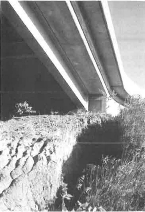
Figure 22. Undesirable side effects of free water escaping through joints.
