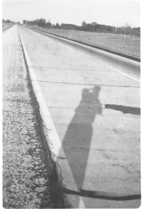
Figure 2. Dowels locked in corrosion with movement coming midslab on a 6-yr-old turnpike.
