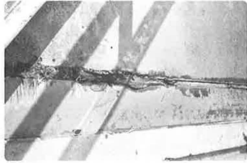
Figure 25. Sliding plate joint seal failure.
