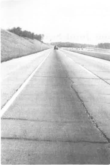
Figure 1. Complete structural failure on a 7-yr-old turnpike.
