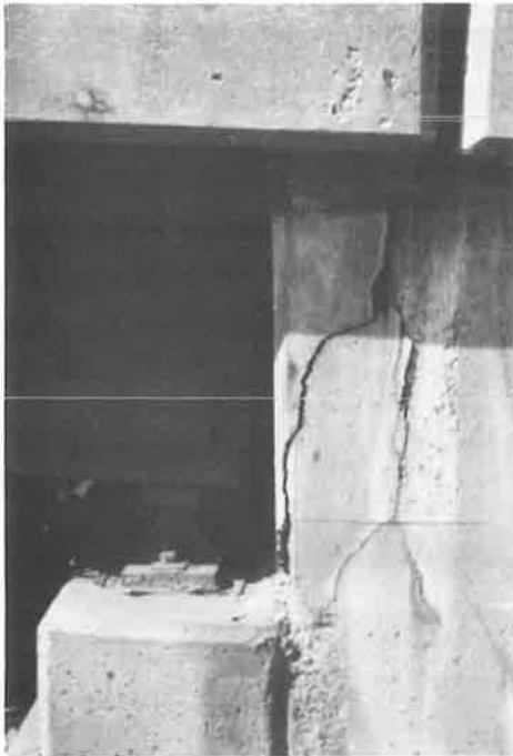
Figure 16. Split back wall on 10-yr-old bridge.
