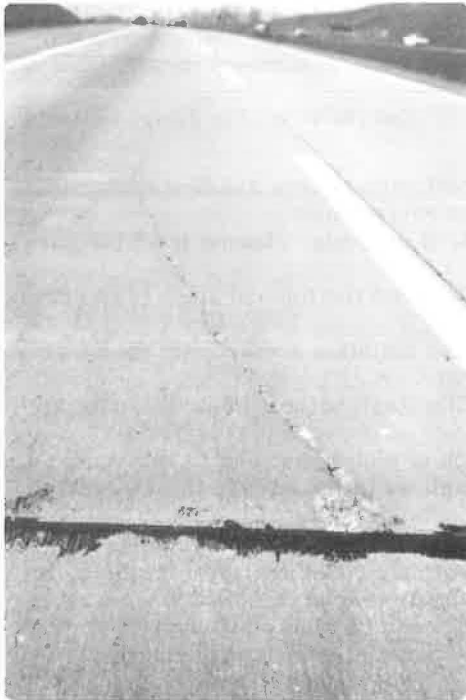
Figure 3. Off-center longitudinal breaking on a 3-yr-old Interstate highway.
