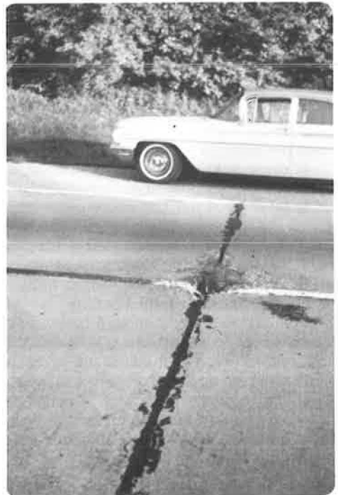
Figure 4. Crushing tends to come first at juncture of transverse and longitudinal joints.
