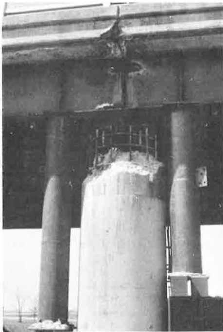
Figure 19. Salt brine corrosion.
