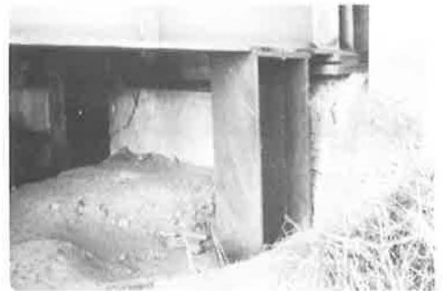
Figure 17. Crushed bearing seat on a 6-yr-old structure.
