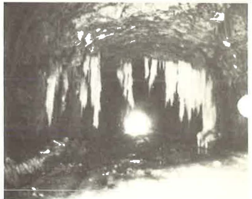
Figure 8. Tunnel near Mile 15.8, Richardson Highway, showing spring seepage.
