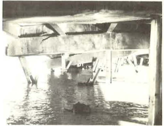
Figure 14. Fractured rail piling beneath Scott Glacier Stream bridge, Copper River Highway.
