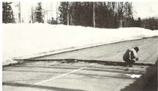
Figure 4. Crack approx. 5 in. wide and 6 ft deep in Richardson Highway near Mile 3, showing vertical displacement.
