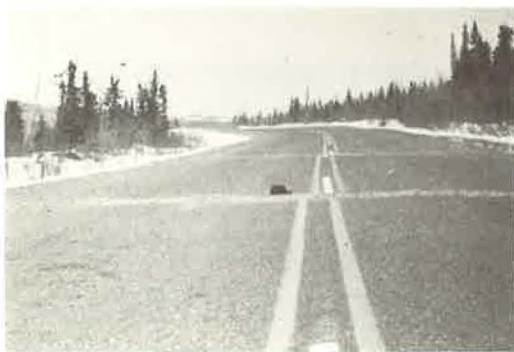
Figure 9. Cracks in Richardson Highway near Mile 73, showing horizontal offset of centerline.
