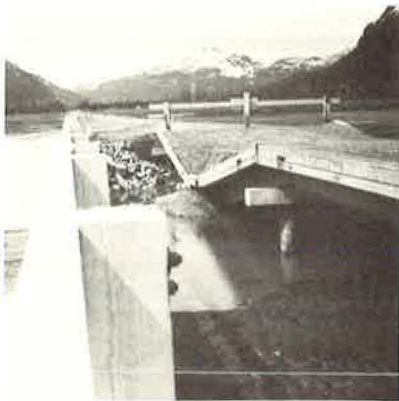
Figure 15. Loss of entire bent supported by timber piling; one of Scott Glacier Stream bridges.
