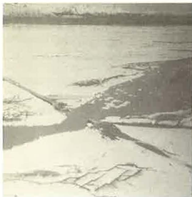
Figure 10. Aerial view of 35 Mile bridge on Copper River Highway with four spans totally destroyed; note ground breakage and evidence of sand ejection.
