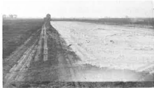
Figure 12. Completed spread from one load of bulk lime directly down runway edge (note uniformity of spread).
