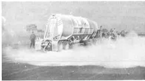
Figure 11. Spreading bulk lime with a long sweep discharge elbow attached to bulk transport; only a slight amount of dusting and air-borne lime.
