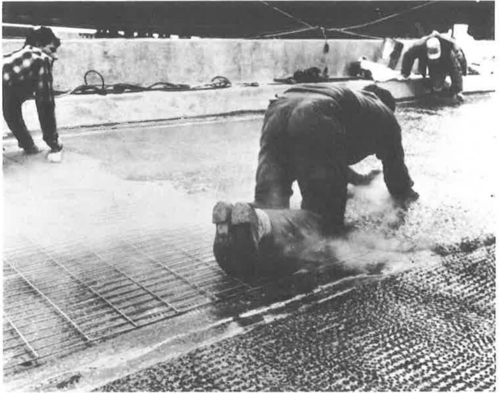
Figure 9. Laying of mastic asphalt with lower right hand area prepared for installation of wire mesh heating elements.
