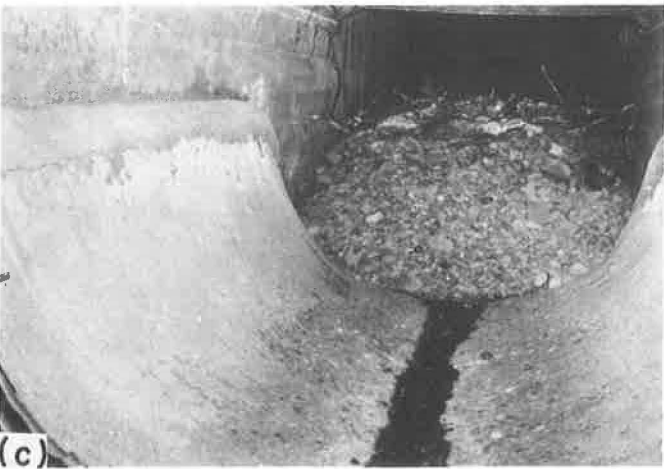
Figure 8. Abrasion test site, IV-SC1-5-C, Sta. 250+25, Bridge No. 37-165: (a) "as built" concrete test section at inlet section of test culvert; (b) appearance of concrete test section after 1.4 yr of service showing severe abrasion; (c) view showing loss of approximately \frac{1}{2} in. of concrete in the concrete test section at the outlet (note deposit of culvert).
