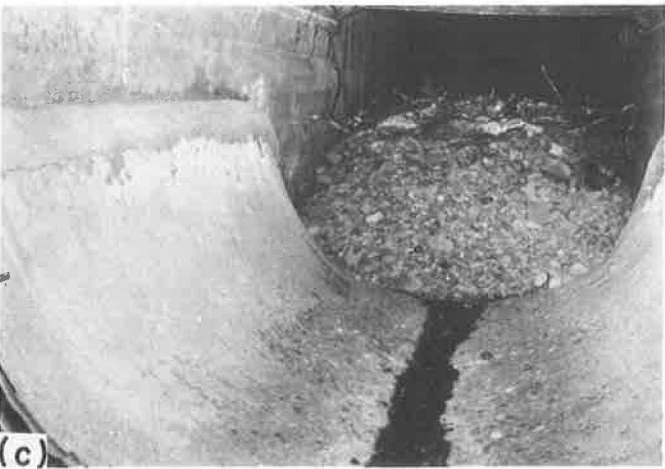
Figure 8. Abrasion test site, IV-SC1-5-C, Sta. 250+25, Bridge No. 37-165: (a) "as built" concrete test section at inlet section of test culvert; (b) appearance of concrete test section after 1.4 yr of service showing severe abrasion; (c) view showing loss of approximately \frac{1}{2} in. of concrete in the concrete test section at the outlet (note deposit of culvert).
