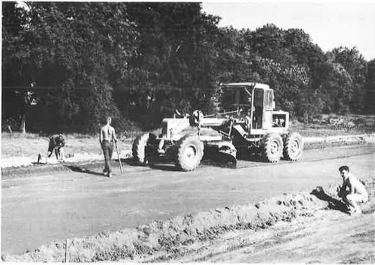
Figure 1. String line crew determining amount to be cut or filled and signalling to grader operator.
