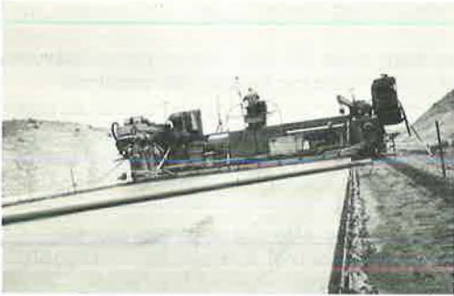
Figure 13. Twenty-four-foot Guntert-Zimmerman paver operating in California with pipe drag in lieu of conventional hand finishing.
