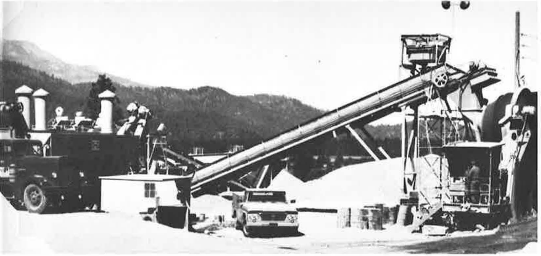
Figure 7. Low-profile central mix plant.
