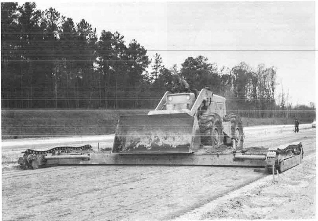
Figure 5. Subgrade planer, running in prepared trenches, cutting central portion of subbase to grade.
