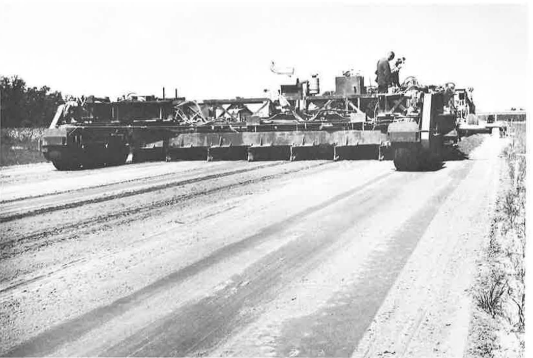
Figure 7. Self-propelled subgrading machine, built by paving contractor, supported on three large wheels in tandem at each corner to provide additional flotation in unstable sands.
