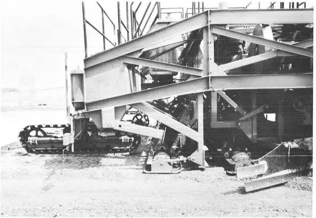
Figure 11. Wire-controlled machine spreading, from windrow, striking off to loose grade, and partially compacting subbase material.
