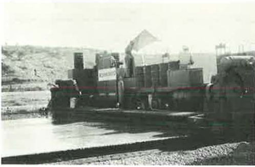
Figure 11. Owl Slip-Form Concrete Co. paving I-10 in southern California with 36-ft Guntert-Zimmerman paver.
