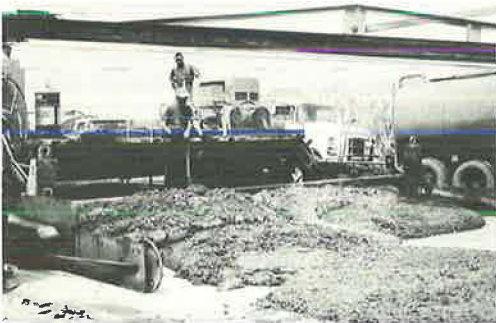
Figure 2. Koehring dual-drum and tribatch mixers placing concrete in front of first slip-form paver on I-40.
