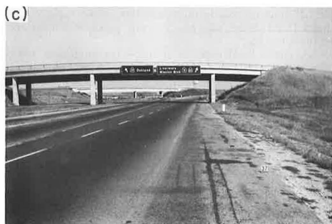
Figure 4. (a) Clear, firm roadside; (b) no pier at shoulder edge (but with sign pole); and (c) pier at shoulder edge.
