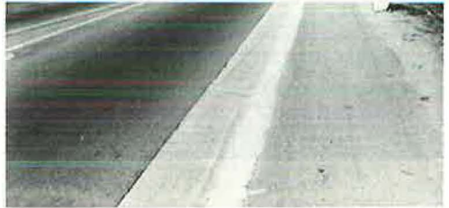
Figure 20. On-ramps, section 23, showing lack of merging distance.
