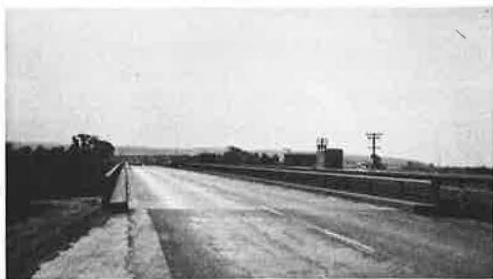
Figure 32. Otay River bridge, showing northbound lanes looking south; guardrail on other end of bridge.
