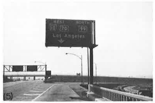
Figure 26. Construction of new ramp; southbound on US 91 to westbound on San Bernardino Freeway in Colton.
