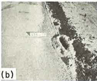
Figure 1. (a) Pavement pumping; ejection of mud and water; (b) blowing; ejection of sand and water.
