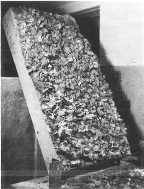
Figure 20. Underside of 4-ft by 2-ft by 6-in. slab bonded to water-bound macadam base (dry) after test.
