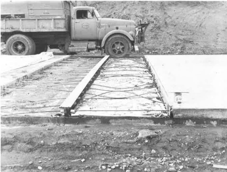
Figure 28. Slack cables protruding from ends of slabs.
