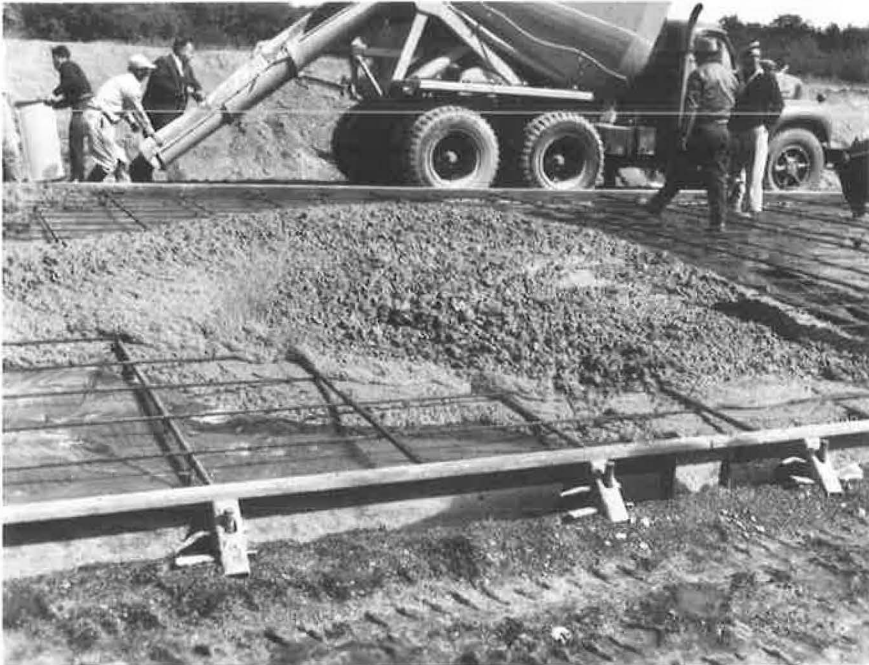
Figure 13. Placement of high-slump concrete, showing considerable segregation.
