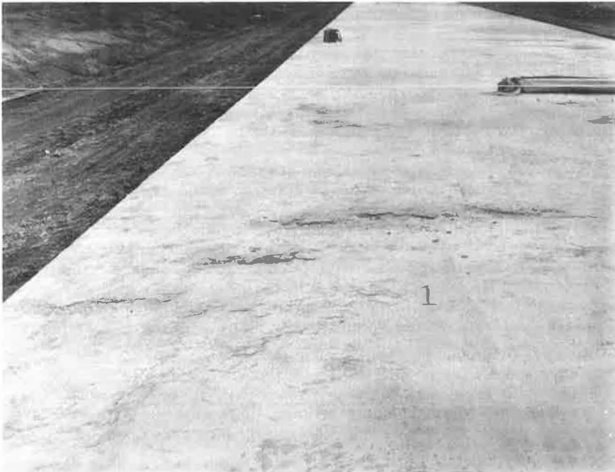
Figure 15. Surface cracks in slab I, day after completion.
