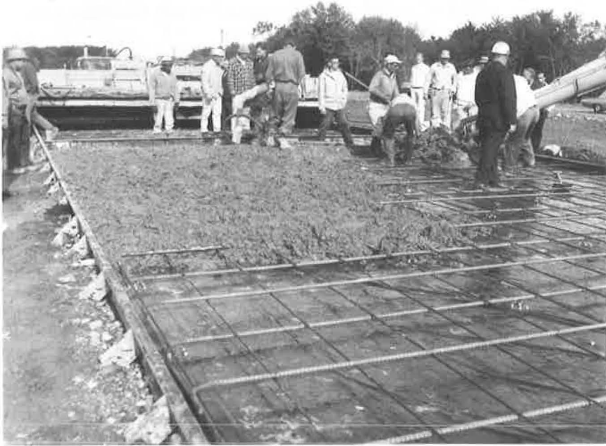
Figure 12. Placement of first load of concrete, showing inadequate slump.
