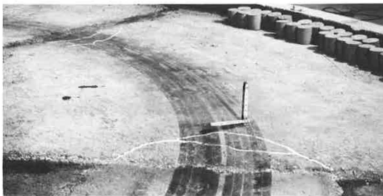
Figure 28. Crack patterns observed on test pavement 2 of test set IV after 175 load applications with white paint applied to outline location of cracks.
