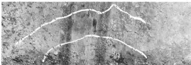
Figure 29. Crack patterns observed on test pavement 6 after 175 load applications, with white paint applied to outline location of cracks.
