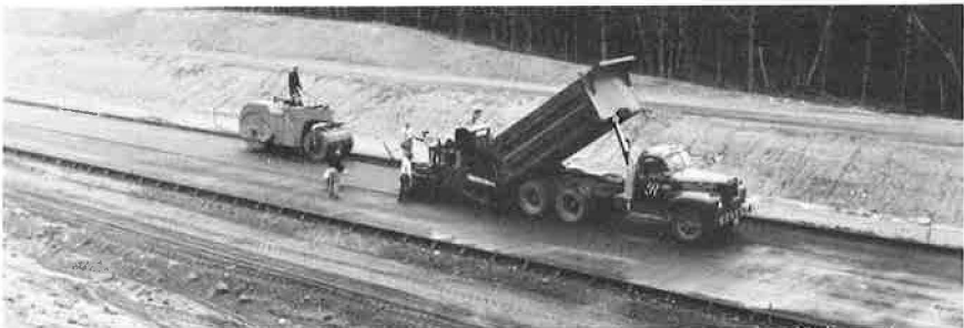
Figure 3. Backfilling forms with 2-in. layer of trap rock screenings and 1-in. layer of dense-graded bituminous concrete.
