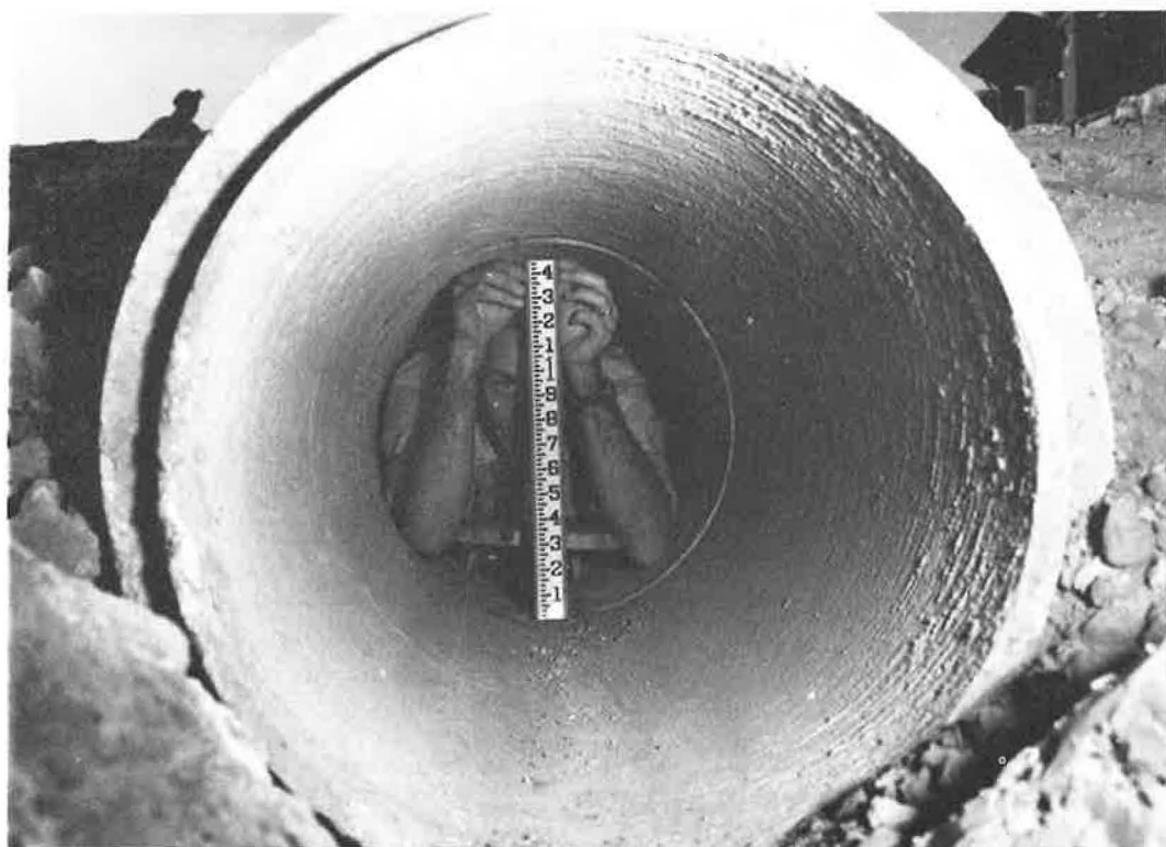
Figure 7. Short section of level rod used in conjunction with transit to measure culvert settlement.
