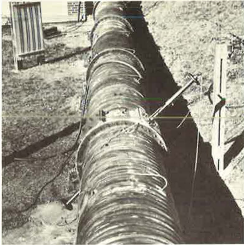
Figure 3. Piezometers and velocity probes.
