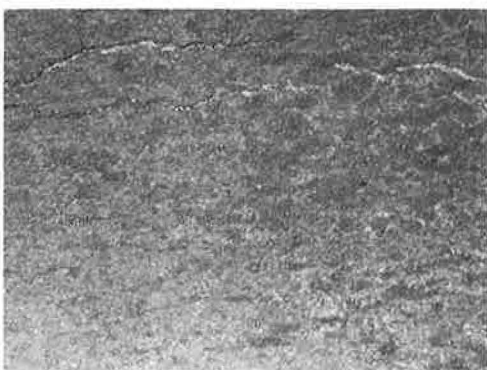
Figure 12. Typical pavement failure.
