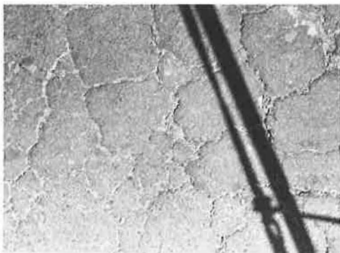
Figure 9. Typical pavement failure.
