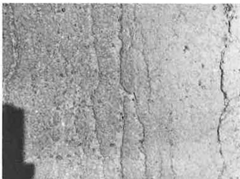
Figure 10. Typical pavement failure.
