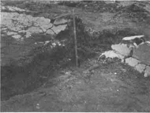
Plastic failure of base and subbase—unstable base and subbase materials.
