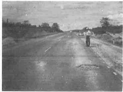
Alligator cracks and holes spreading along pavement.
