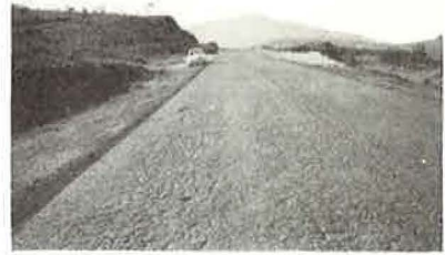
Pavement fatigue failure—alligator cracks on both inner and outer wheelpaths.
