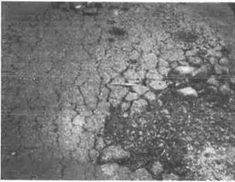
Alligator cracks and hole formation.
