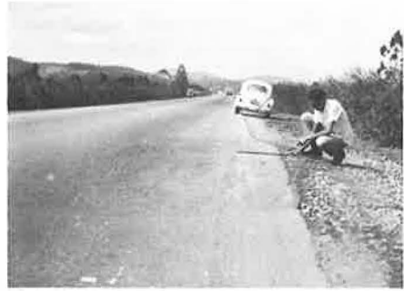
Plastic failure of subgrade—poor foundation, underdesigned pavement.
