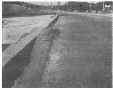
Plastic failure of asphalt surfacing—unstable bituminous mixture.
