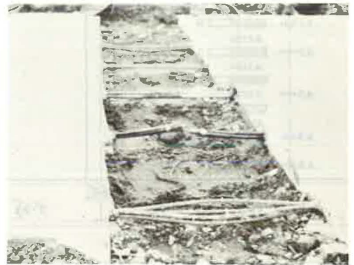
Figure 4. Ungrouted tendon severed.
