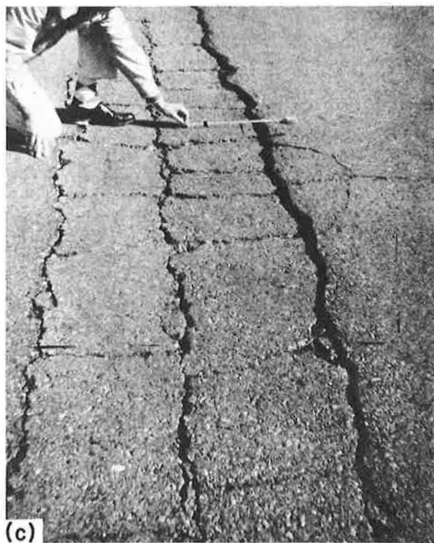
Figure 4. Typical progressive deterioration from shoulder cracking: (a) early shoulder cracking; (b) progressive cracking into driving lane; and (c) ultimate failure.
