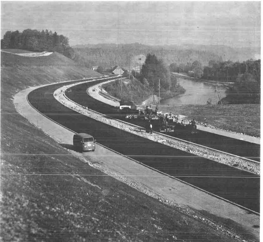
Figure 17. Two pavers equipped with electronic screed control, working in echelon, on Swiss highway N 1 Berne-Zurich.
