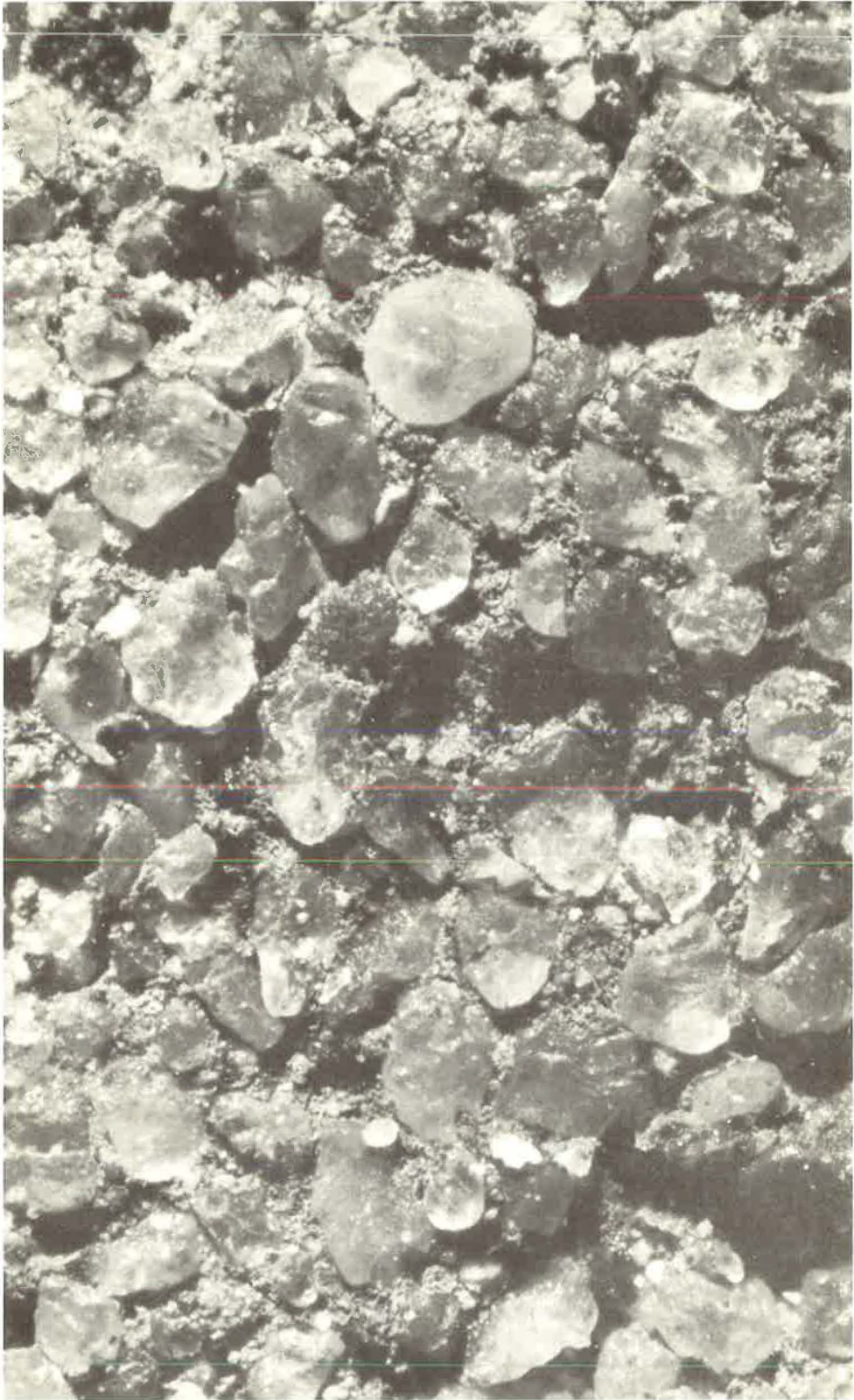
Figure 4. Leaching of weathered mortar from the untrafficked surface of sand asphalt—magnified view after ten months' exposure on laboratory roof.
