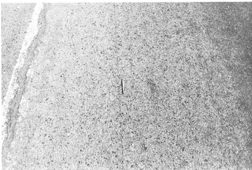
Figure 15. Condition of bituminous surface at typical intersection.
