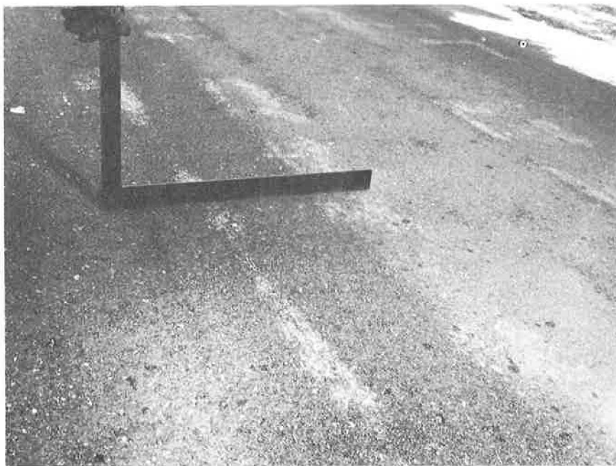
Figure 8. Surface of bituminous pavement after 210 normal stops.
