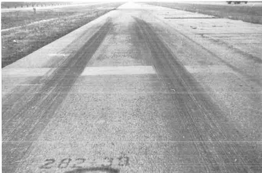
Figure 9. Bituminous-concrete surface after application of 175 normal stops followed by 25 emergency stops.
