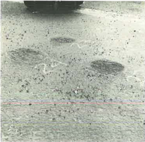
Figure 13. Test nos. 22, 23, 24 (asphaltic-concrete pavement): stud scour depth 0.15 in. (no. 22), plain snow tire scour depth, 0.14 in., maximum; chain scour depth, 0.50 in., maximum (no. 24).
