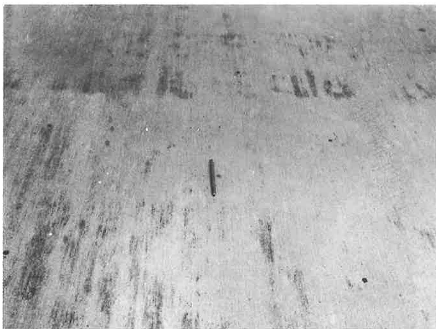
Figure 4. Surface of concrete after 210 normal stops.
