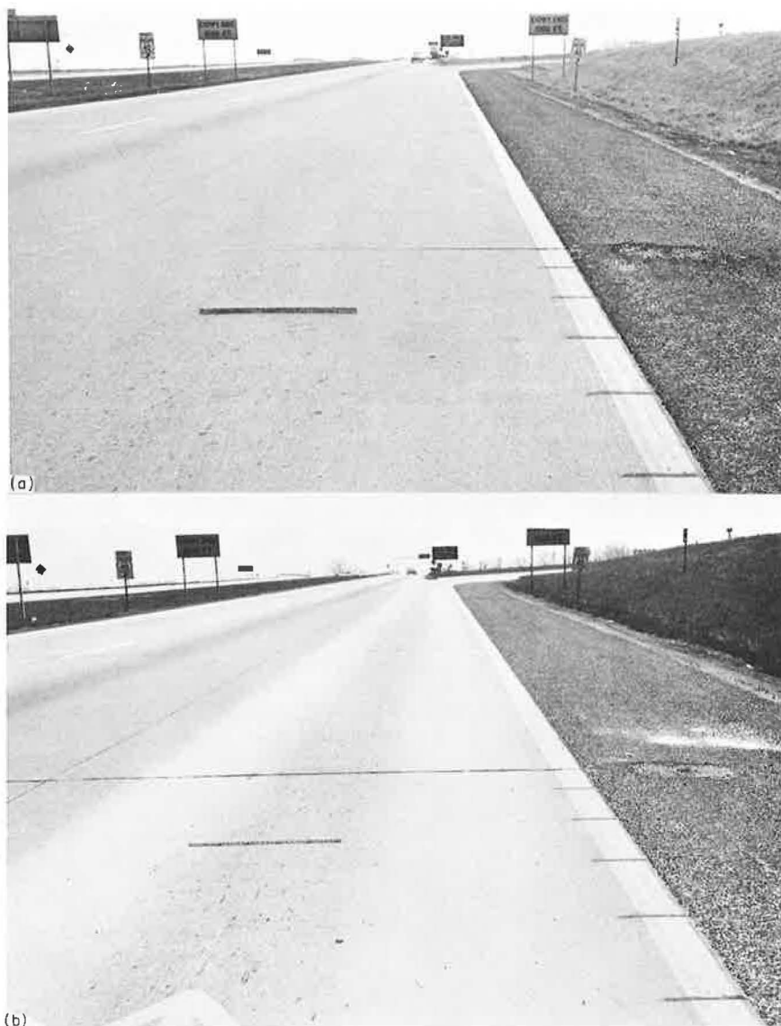
Figure 11. Truck test loop, rigid pavement (a) before test and (b) after test, Md. 7 and Baltimore Beltway.
