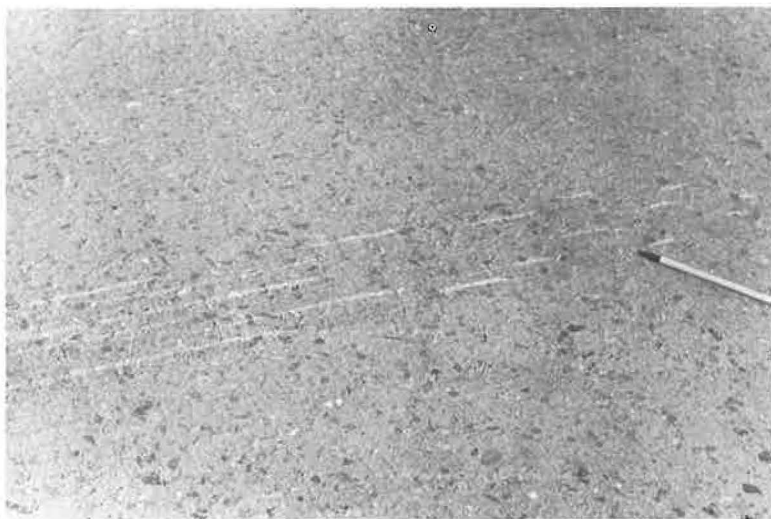
Figure 6. Skid marks on concrete pavement.
