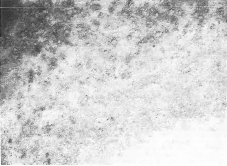
Figure 13. Gray transition zone adjoining rusted area in Figure 12, pits, blisters and rust nodules in aluminum coating (surface 2 X).
