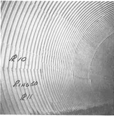
Figure 9. Failure of longitudinal seam allowed plate slippage.
