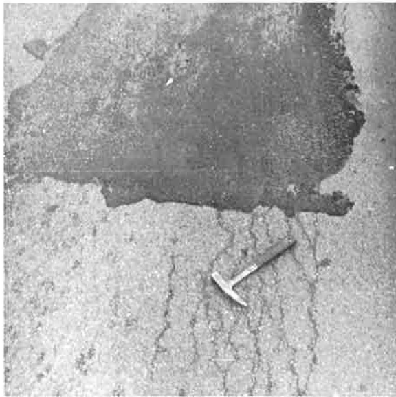
Figure 4. Test panel No. 9 (in background) showing arrest of cracking.
