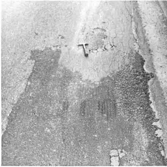
Figure 3. Test panel No. 9 showing superior condition of rubber-asphalt repair.
