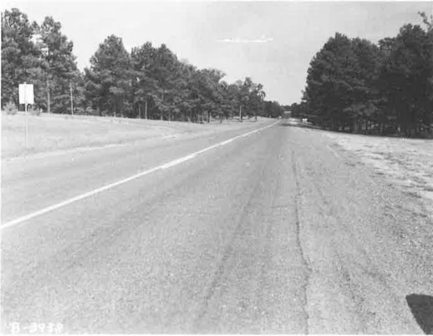
Figure 60. Type F cover aggregate in service three months, 1500 vpd, US 190.
