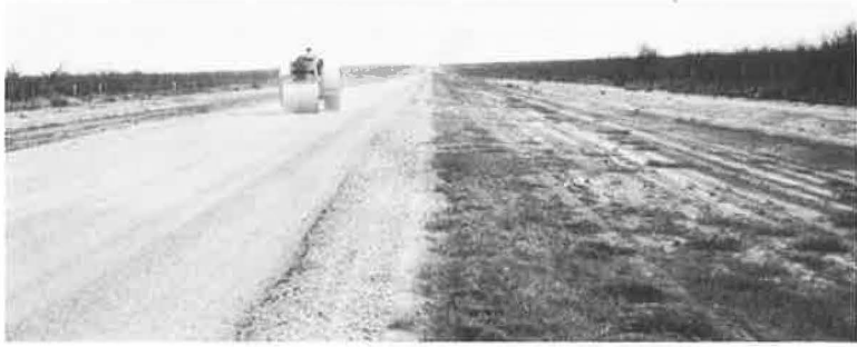
Figure 53. Experimental section proves that the use of steel flat wheel roller is not advisable.
