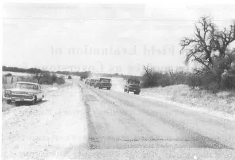
Figure 1. Old surface has variable demand for asphalt from point to point.
