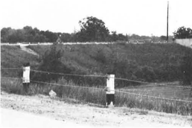
Figure 22. Steep slope and inadequate guardrail adjacent to expressway.
