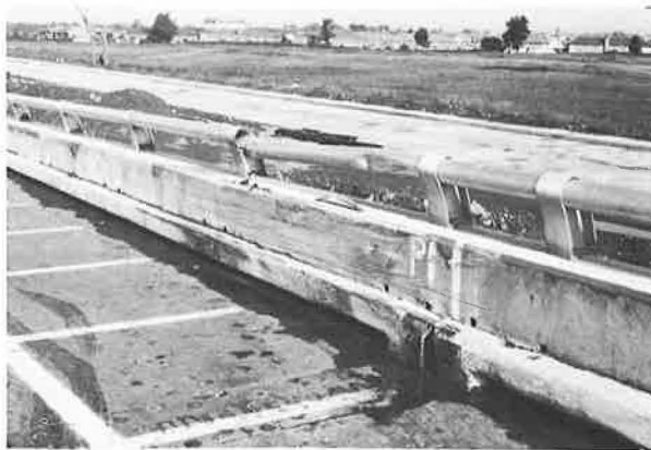
Figure 21. Damages to guide rail model H after the three tests.
