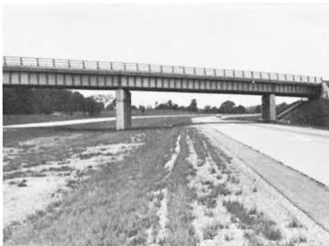
Figure 27. Unprotected bridge abutment—a definite hazard on expressways.
