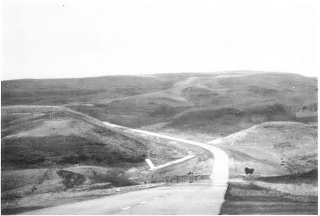
Figure 21. Because the vertical curve is too short, the left edge of the pavement forms a V at the bottom of the hill.
