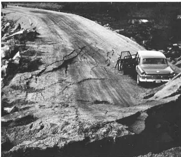
Figure 6. Collapsed section immediately after failure looking north.
