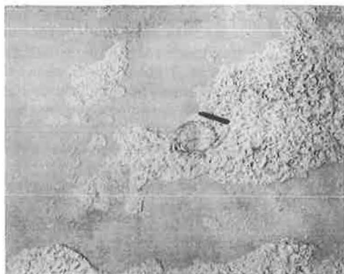
Figure 1. Bridge deck deterioration.
