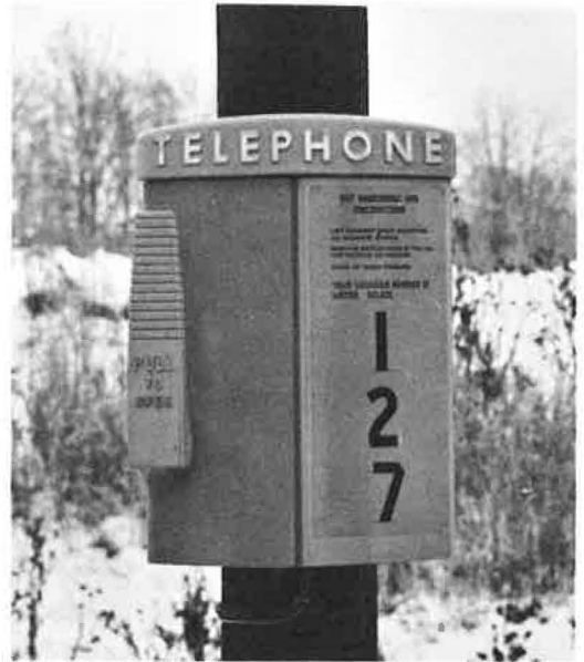
Figure 3. Call box of the emergency telephone system.
