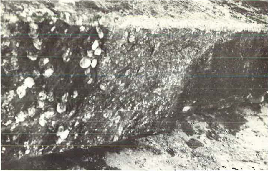
Figure 4. Appearance after removed pile. Note line of demarcation between exposure to free water and mud immersion.
