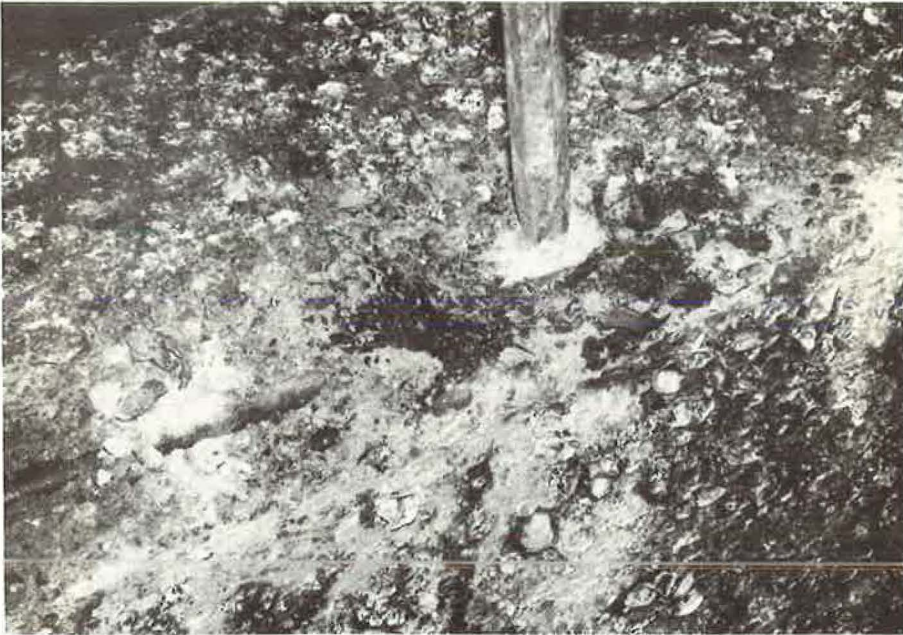
Figure 5. Removing concrete with jackhammer. Note rust stain (dark area) immediately adjacent to bit of jackhammer.
