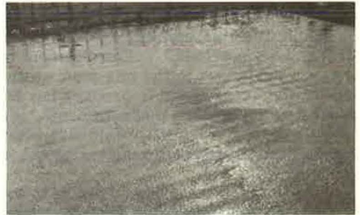
Figure 20. Excessive bleed water.
