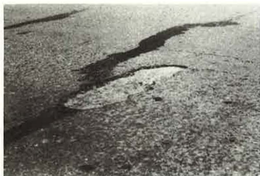
Figure 6. Example of a pothole.
