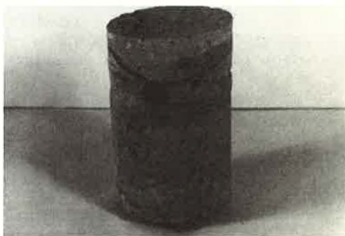
Figure 5. Core showing a fracture plane at the top reinforcing steel.
