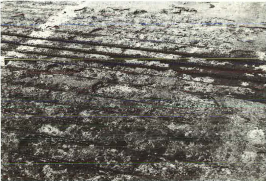
Figure 10. Deteriorated surface showing exposed reinforcing bars; the steel is close to the top surface of the deck.
