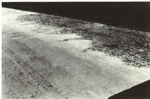
Figure 7. Severe surface mortar deterioration; as much as 2 in. of the deck has eroded away.
