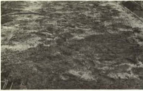
Figure 21. Excessive walking in the fresh concrete.
