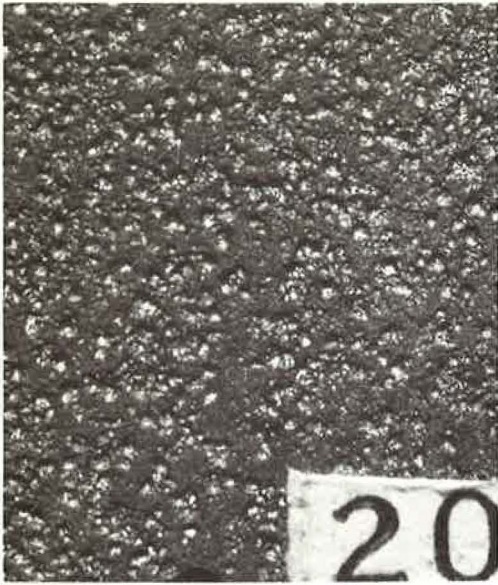
Figure 37. Example of light pitting in exposed portion of coupon—coupon exposed for 12 months in Test Rig No. 2.
