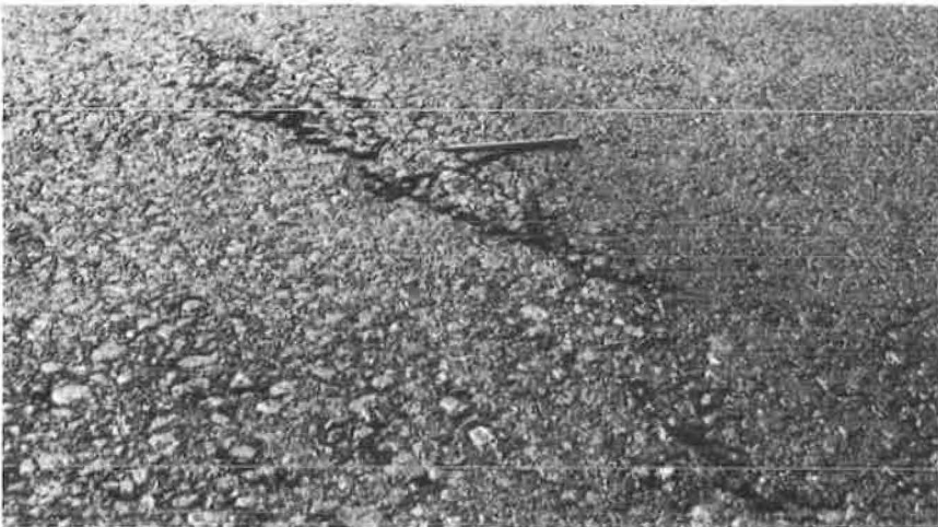
Figure 9. Excessive shoving of binder course.
