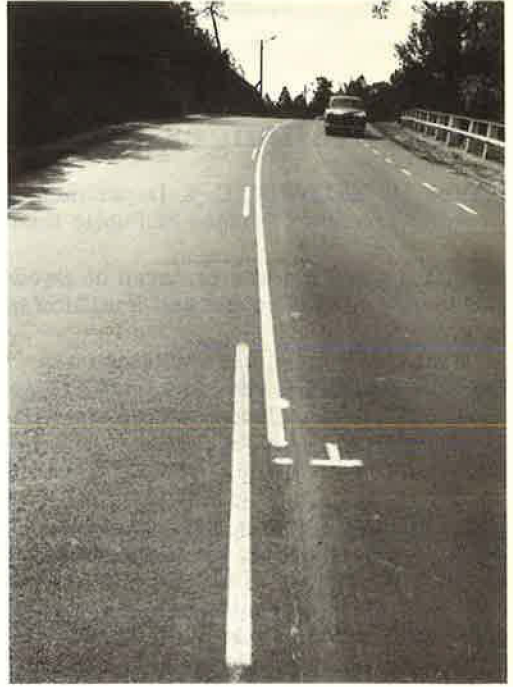
Figure 2. New pavement markings installed before the changeover while left-hand traffic was still operating.
