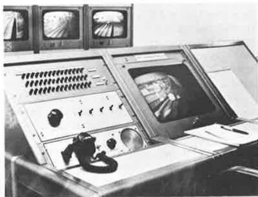
Figure 12. Monitor arrangement in central control center.
