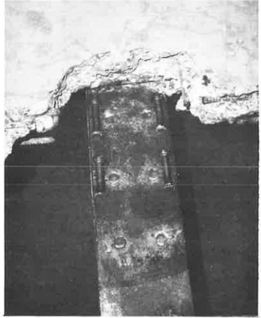
Figure 15. Studs at the east inflection point of beam CC-1F after fatigue testing.
