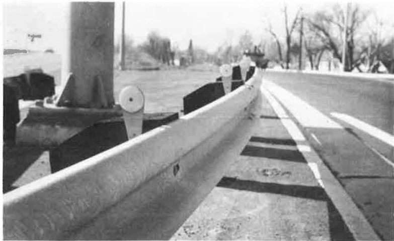
Figure 9. Metal beam guardrail reflector assemblies.
