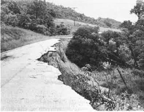
Figure 1. Slide of a highway embankment weakened by saturation caused by a clogged culvert.
