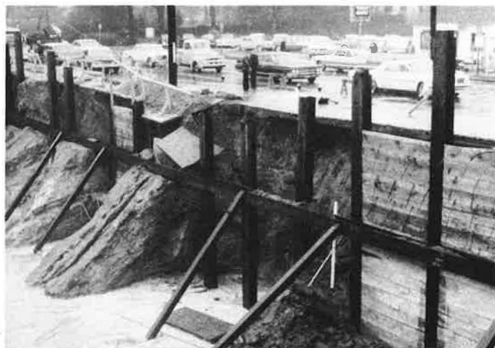
Figure 2. Failure of soil face behind soldier piles where installation of the lagging had been delayed. The dropout destroyed the sidewalk and an 18-inch water main and undermined a 6-lane pavement.
