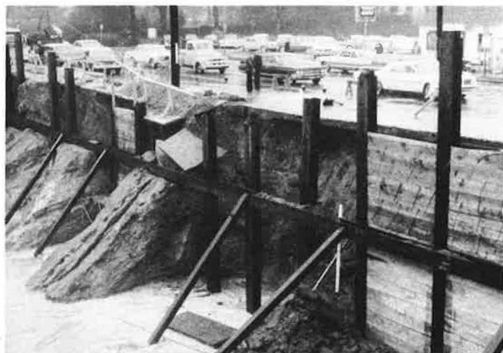
Figure 2. Failure of soil face behind soldier piles where installation of the lagging had been delayed. The dropout destroyed the sidewalk and an 18-inch water main and undermined a 6-lane pavement.
