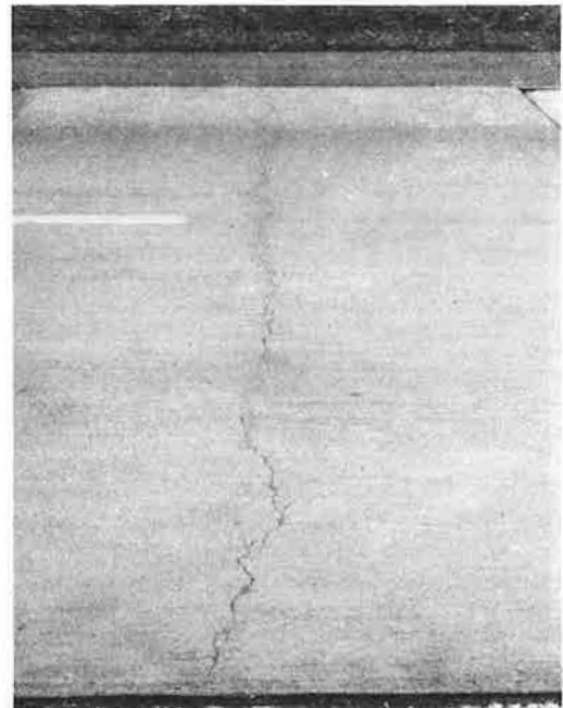
Figure 34. Transverse crack in filler block 3 approximately at mid-length of the block.
