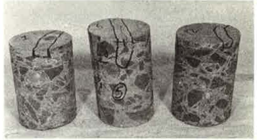
Figure 12. Cores taken at partial transverse cracks; core numbers 1, 5, and 12 taken in slabs I, II, and III respectively, January 1966.
