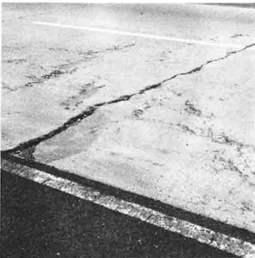
Figure 29. Distressed area of slab; width of spall, 3 to 6 in.; at median edge, 12-in. steel not visible.
