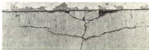
Figure 26. Close-up of cracking in Figure 25, April 1964.
