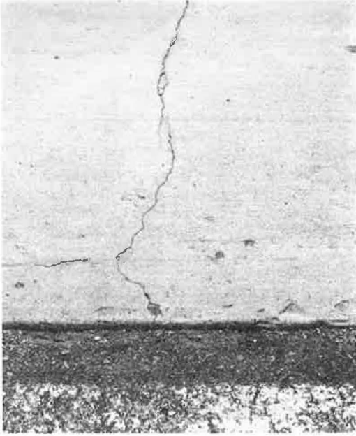
Figure 31. Close-up of area in Figure 30 showing longitudinal edge crack.
