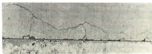
Figure 25. Longitudinal and semicircular cracks, same location as Figure 24, April 1964.
