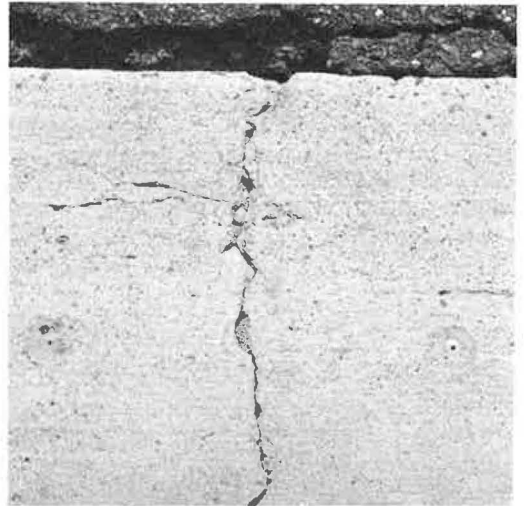
Figure 28. Slab I—gage plug instrumentation at a partial transverse crack, mid-length of slab; longitudinal edge crack in upper center of photo.
