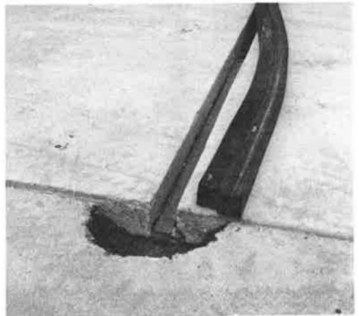
Figure 6. Joint 3—seal ready for placement; note the redwood strips used for support.
