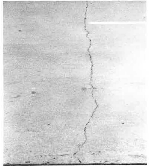
Figure 30. Transverse crack 15 ft south of distress in Figure 29; minor spalling, crack tight.
