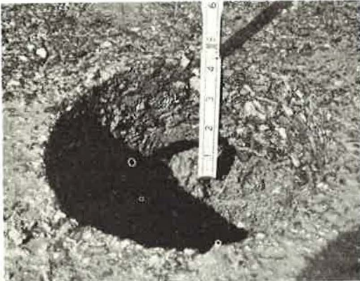
Figure 6. Core hole with void under AC surfacing.
