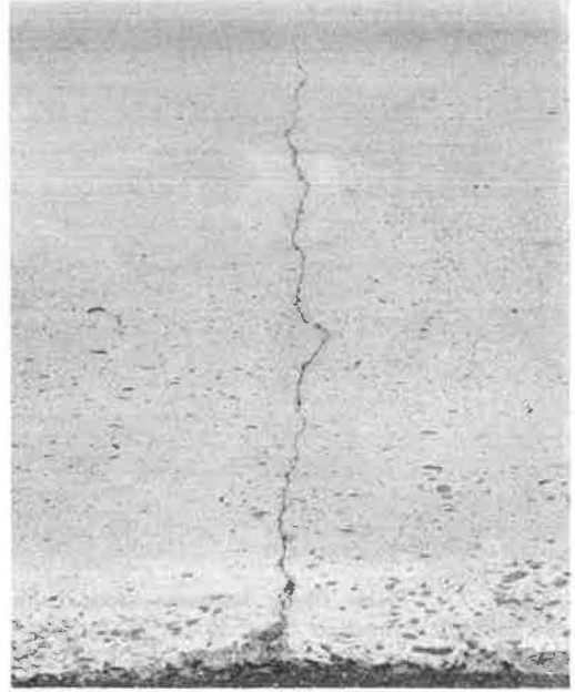
Figure 32. Transverse crack in slab II; rust spots on surface of pavement at crack.
