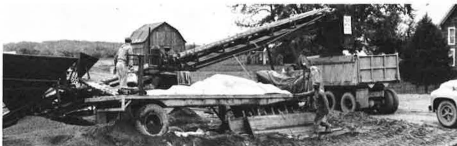
Figure 4b. Conveyor and baffle box for mixing aggregate, fines, and salt.
