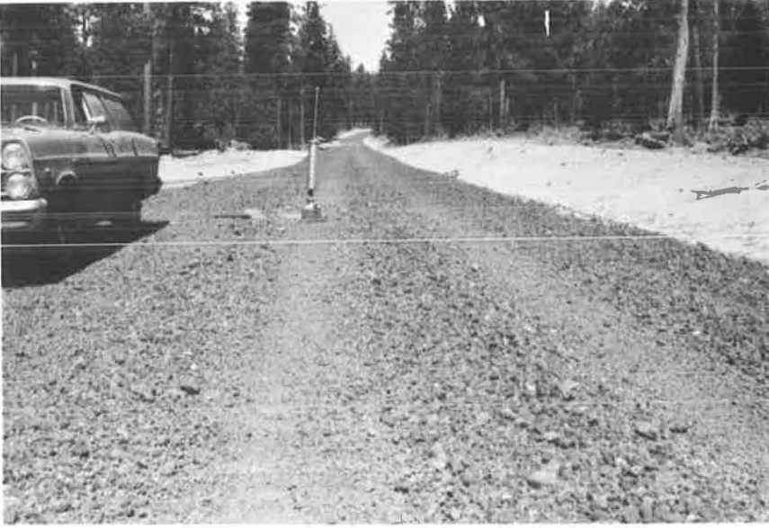
Figure 2. Kirk Road, Northeast of Chiloquin, Oregon: Rough surface contains black, uniformly graded cinders (PI = 2.1).
