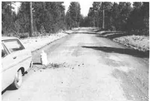
Figure 4. Road 33061 (East-West) West of Chiloquin, Oregon (PV = 3.2, PI = 3.3).
