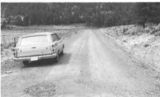
Figure 5. Road 379 (Fishhole) South of Bly, Oregon (PV = 4.3, PI = 4.1).
