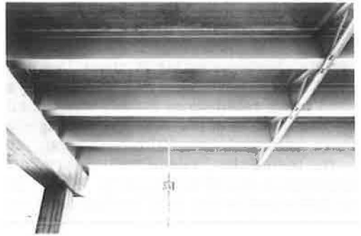
Figure 3. System 14—Inorganic zinc and silicate primer, post-cure type, and vinyl primers and vinyl finish coat.
