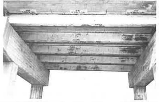
Figure 1. Panel 8N—Zinc chromate primer and No. 5 aluminum finish coat; panel 9N—red lead and oil primer and No. 5 aluminum finish coat; panel 10N—red lead and oil and aluminum finish coat.
