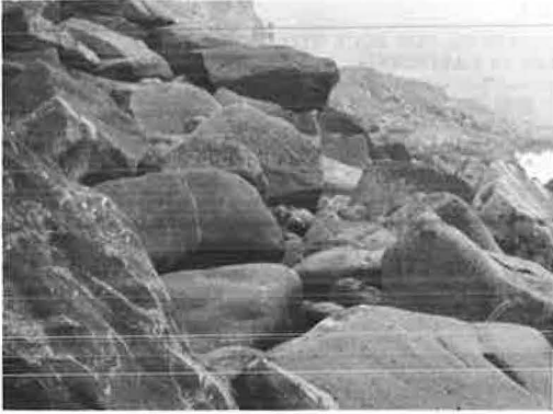
Figure 1. Good installation of sedimentary and igneous rocks. Severe rounding caused by wave action.
