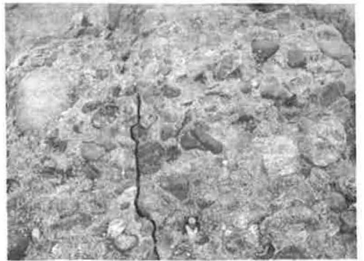
Figure 6. Unsatisfactory sedimentary rock.
