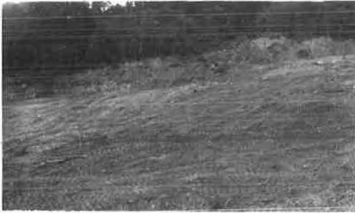
Figure 7. West scarp of the 1967 Tremont slide showing scar on old landslide debris. Bedrock visible in middle background along old landslide scar, dips about 10 degrees to left. View is northwestward (Deen and Havens, 2).
