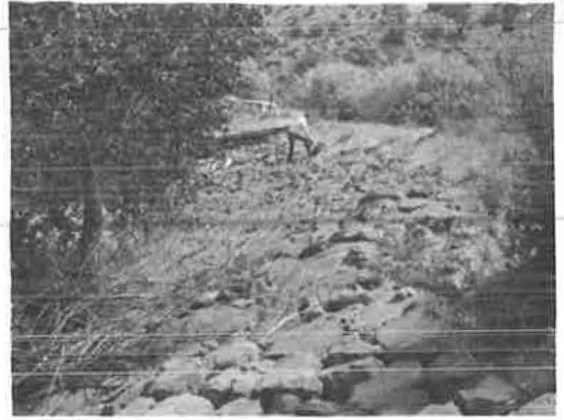
Figure 2. Good installation of sedimentary rock in place for 23 years. This material does not comply with the Standard Specifications.
