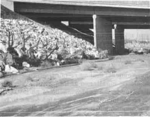
Figure 3. Unsatisfactory installation of good igneous rock.
