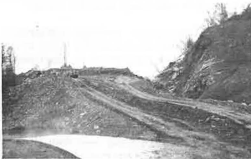
Figure 9. Southwestward view of deep roadcut west of Wallins Creek quadrangle where sandstone, shale, and siltstone in lower part of Breathitt Group slid down a dip slope into the excavation.
