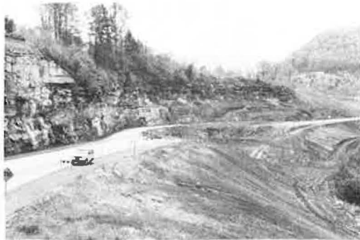
Figure 6. Strata in lower, unstable part of Breathitt Group at Church slide. Roadbed taken out by 1969 slide, rebuilt on strata that continue intermittent down-dip movement toward observer.
