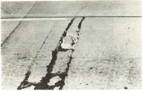
Figure 20. Typical failure on I-55 in Madison County.
