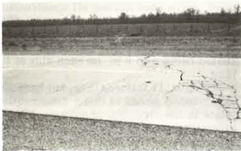
Figure 22. Failure on top of lapped splices on US-82 in Leflore County.
