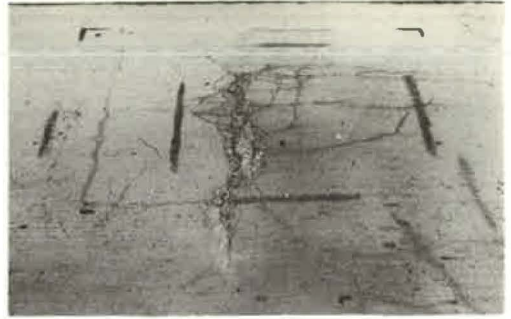
Figure 21. Defective area on I-59 in Pearl River County.
