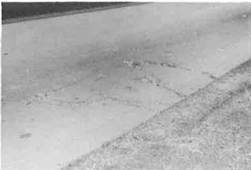
Figure 25. Failure caused by embankment settlement on I-20 in Hinds County.
