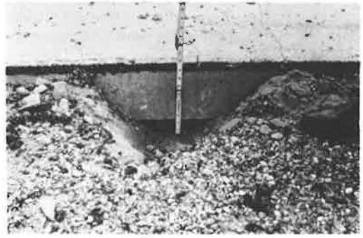
Figure 24. Void spaces of 2.5 in. between pavement and subgrade on I-55 in Carroll County.
