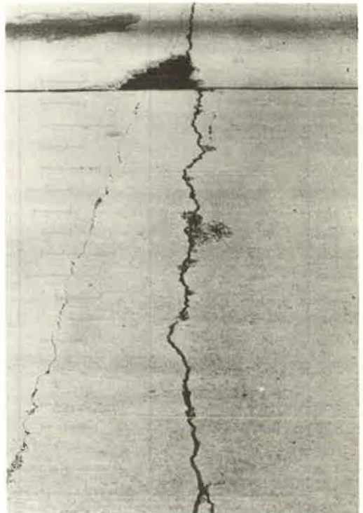
Figure 16. Extra-wide cracks on I-59 in Jones County.
