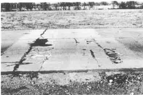
Figure 34. Patch poured in morning 8 months after repair on I-55 in Madison County.
