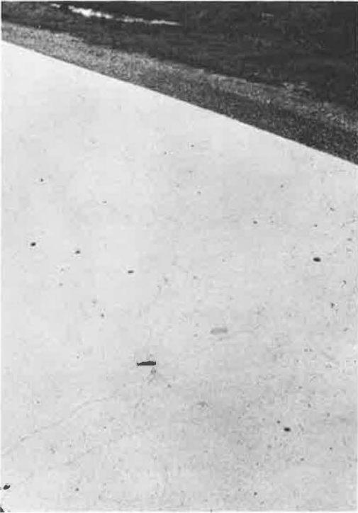
Figure 23. Transverse and diagonal cracks on I-55 in Carroll County.
