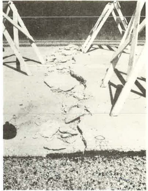
Figure 26. Failure on I-55 in Copiah County.
