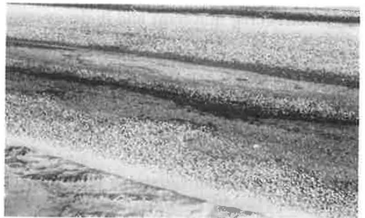
Figure 4. Extreme wear of bituminous mixture along the wheel track.
