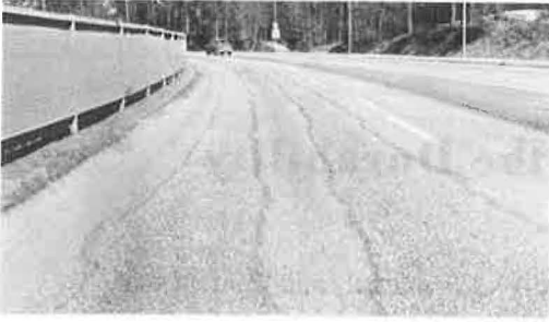
Figure 1. Premature wear by studded tires of pavements submitted to traffic of high density.
