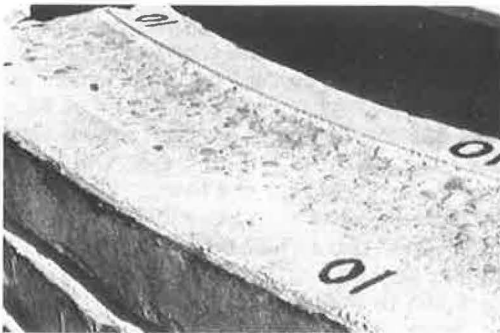
Figure 6. Wear of concrete surfacing by studded tires.
