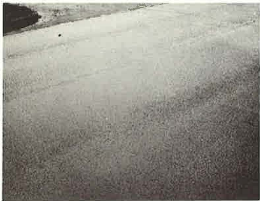
Figure 1. Slippery pavement surface of polished limestone.
