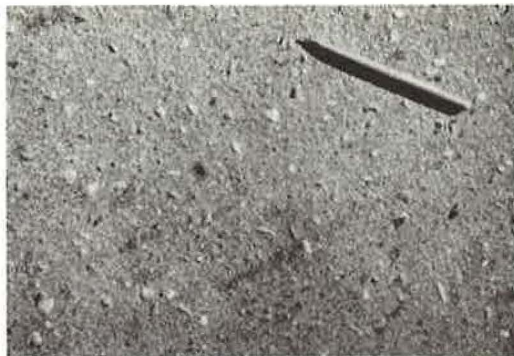
Figure 19. Close-up showing stones sticking out of stone-filled sand asphalt.
