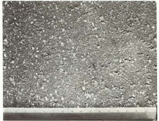
Figure 5. Close-up of sandstone surface 4 years after construction.
