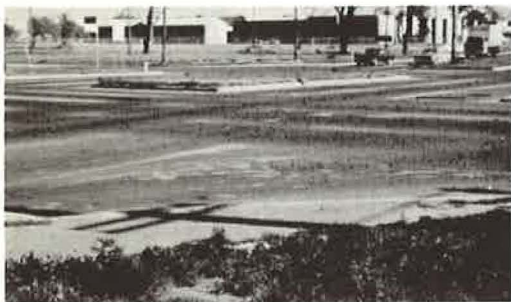
Figure 20. Raveled fillets of sand-asbestos surface 4 years after construction.
