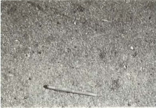
Figure 21. Close-up of sand-asbestos surface 4 years after construction.
