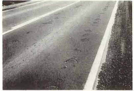
Figure 15. Delamination of sand-asphalt surface 1 year after construction.
