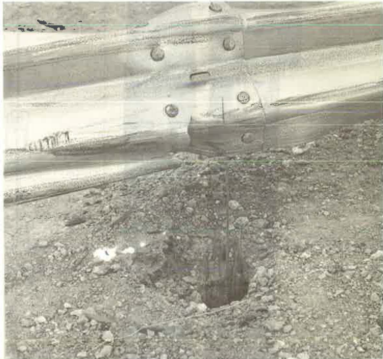
(c) Typical post failure (note tear in rail section)
