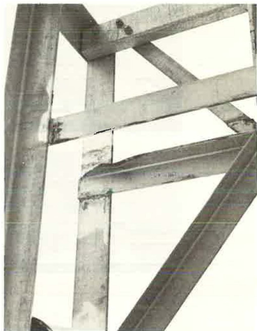
Figure 18. Damage to truss guide angle (Test F).
