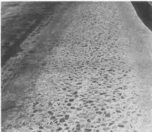
Figure 7. Appearance of concrete surface after 400,000 passes.
